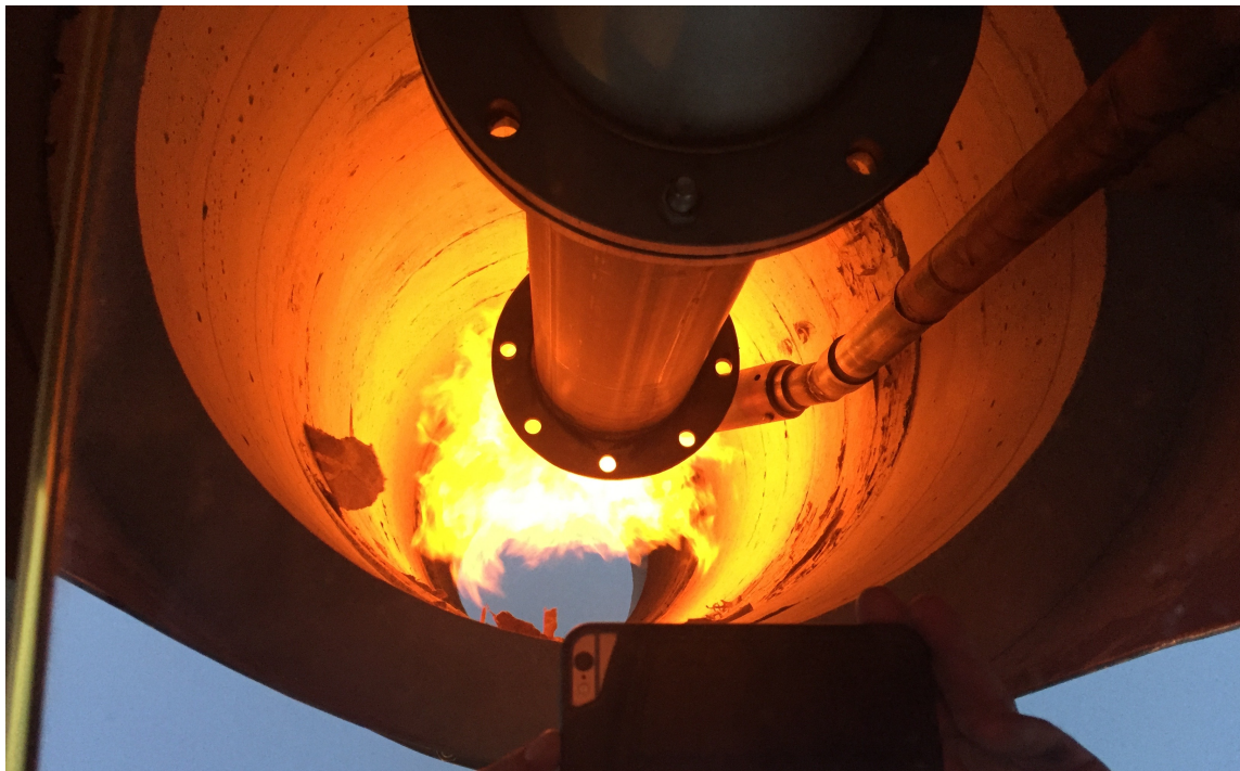
Figure 2.7 The facility will employ an enclosed flare
