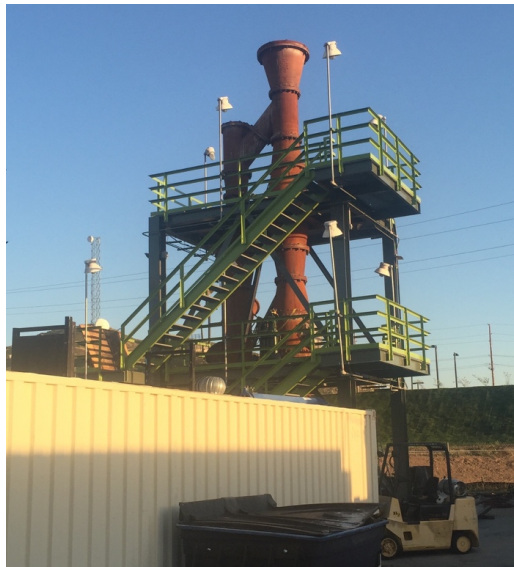
Figure 32: Gasifier (right), Tar-Reformer (left)
