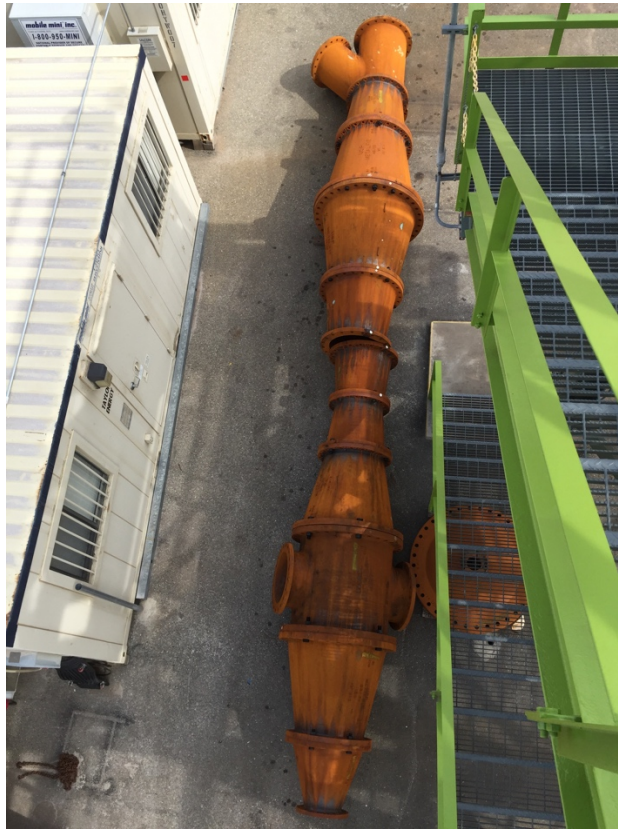
Figure 34: Carbon-steel “spool sections”
