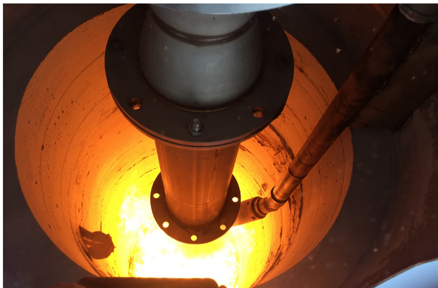
Figure 2.2: The Demonstration Facility will employ an enclosed flare
