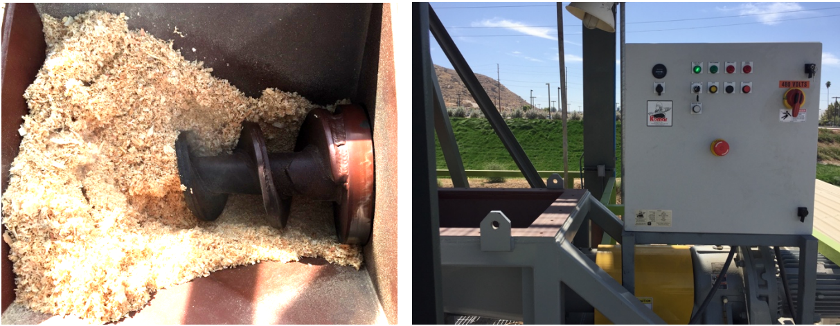
Figure 45: Komar Extrusion Feeder and Variable Frequency Drive that controls the feed-rate
