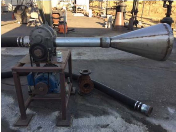
Figure-24. Roots Blower – Powered by a Variable Frequency Drive
