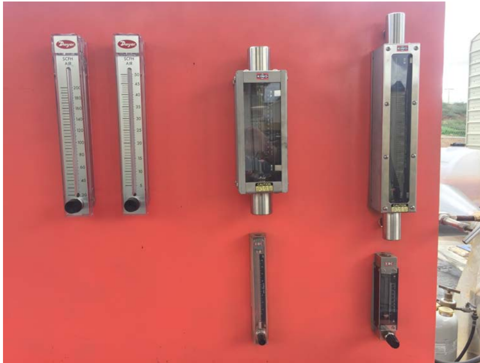
Figure-33. Fuel Measurements
